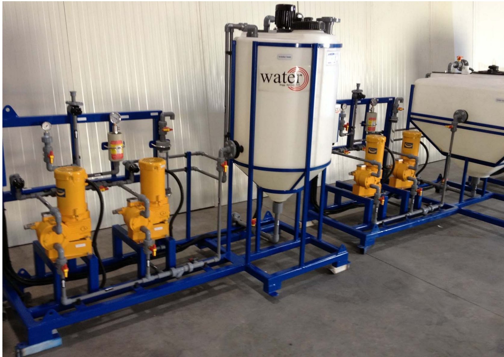
SODIUM HYPOCHLORITE DOSING SYSTEM- (CPVC- HOPPER BOTTOM)
